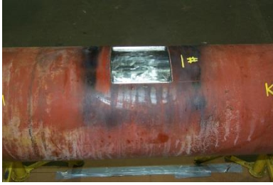
Defect - 6.5" x 6.5" x .300" Deep
